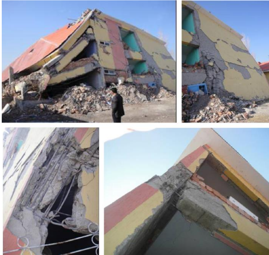
Fig. 6. Photos of the collapsed school building.
