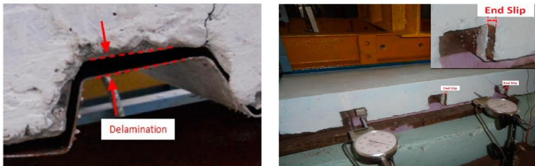
Fig. 2. Delamination and end slip in profiled sheet deck slab (Avudaiappan et al. 2021).
