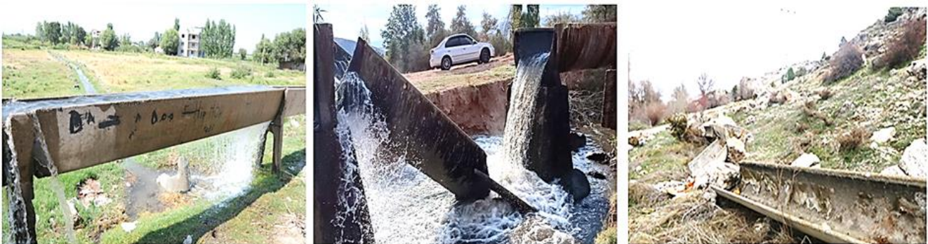
Fig. 2. Damages occurring in various irrigation channel: (a) Manisa; (b) Hasandede/Kırıkale; (c) Kahramanmaraş (URL 2; URL 3).
