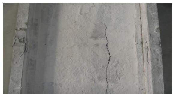
Crack pattern of S10
