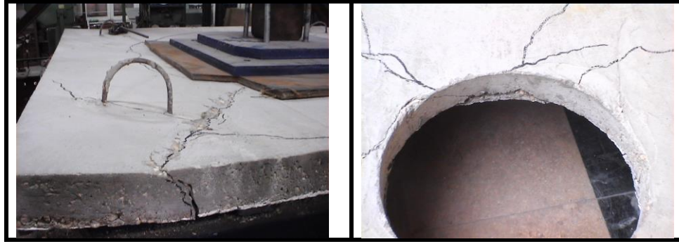
Figure 5 - Shear crack in RM and S_tMC_eCO
