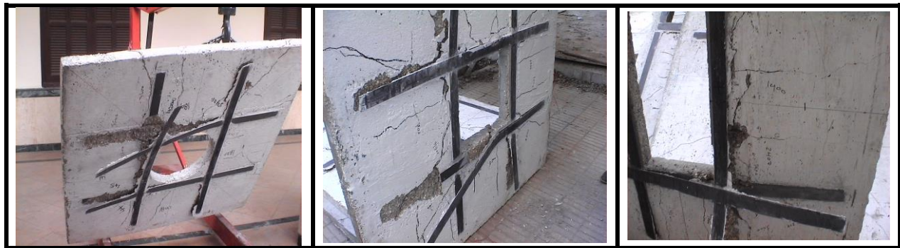
Figure 6 - Failure of epoxy bonding: pull off the concrete cover
